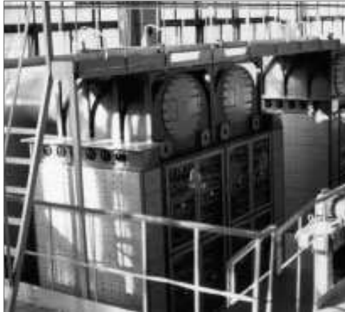
■ Fig 23. UV drinking water plant 405.000 m 3 per day, Tollyaytti (Russia)
